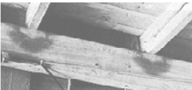
Figure 3. Evidence: rub or swing marks made by roof rats.
